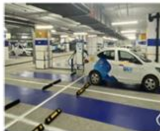
Figure: Charging station of EV fleet
